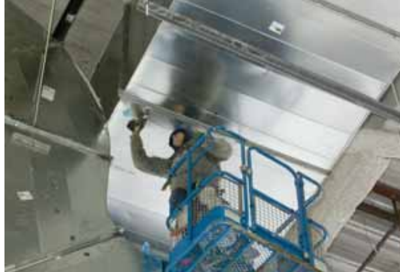
F. E. Moran installer Jim Macis bolts together Quick Flange ductwork frames at the Children’s Memorial Hospital jobsite in Chicago. More than 500,000 pounds of sheet metal are being installed in three tiers of ductwork for the mechanical room of the hospital project.
